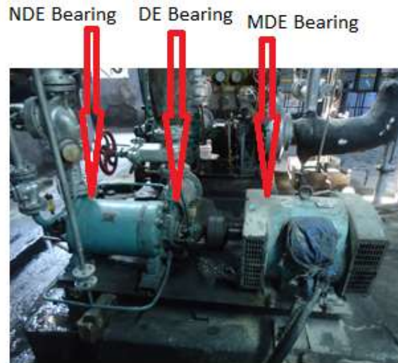
Fig. 2. Photograph of boiler feed pump
